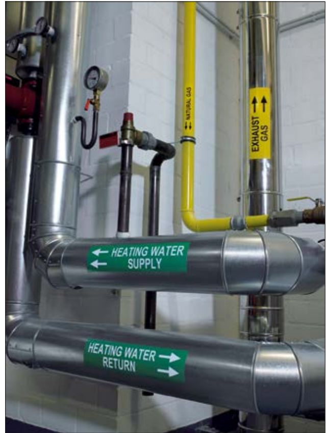
Large and highly visible pipe marking.
