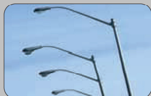
Public lighting Eclairage public
