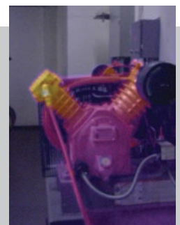
Air Compressor – AutoBlend™ Mode
