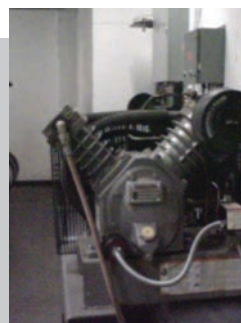
Air Compressor – Full Visible
