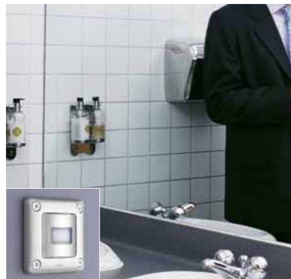
PUBLIC WASHROOMS | Automatic switch
