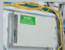
Control Panel Labeling
