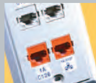
Patch Panel & Faceplates
