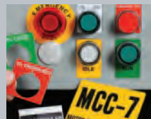
Control Panel Labeling
