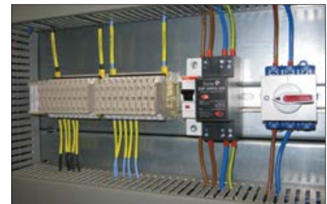
Figure 6. ESP 240 DS-32A installed conveniently in a power distribution cabinet.
